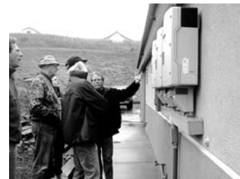
John Parry, SolarWorks founder and owner, explains the new solar system to Fire District supporters.
